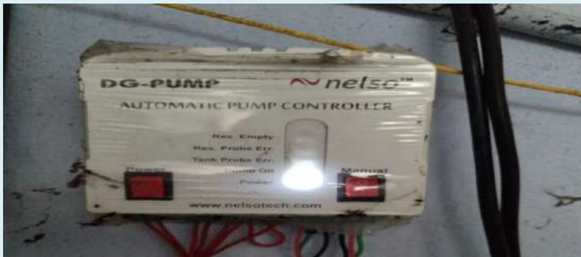
Pump Power Auto Cut and Auto On
